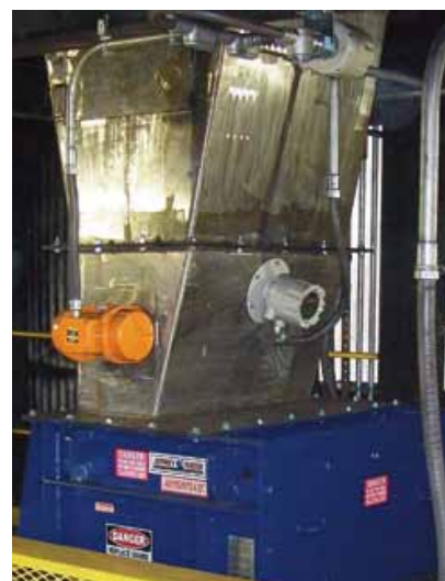
Figure 7. Plugged chute indicator with vibrator.
