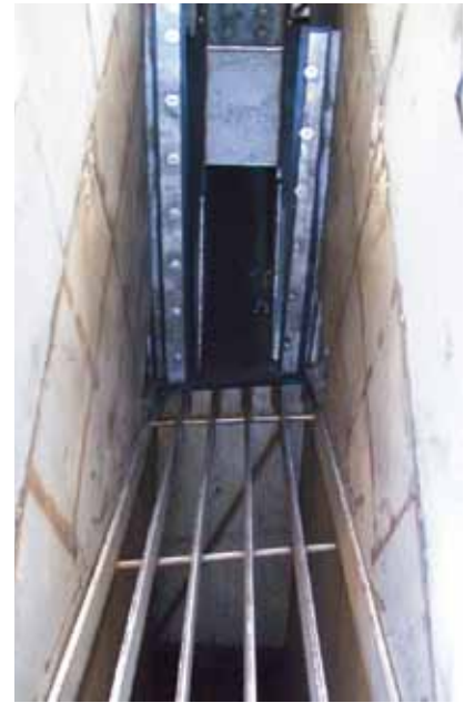
Figure 3. Primary receiving hopper with debris bars.
